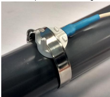
Water temp sensor mounting
